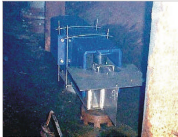
Scale-X™ MFC Installed on the Separation Vessel Water Outlet Standpipe
